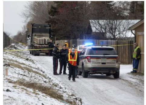
Workplace death: 19-year-old man working on city sound wall project dies after concrete falls on him from truck
